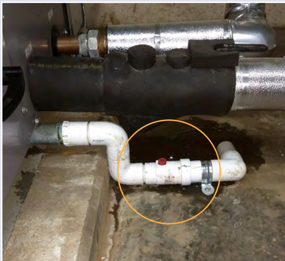
N-Series, commercial mechanical room negative pressure installation.
