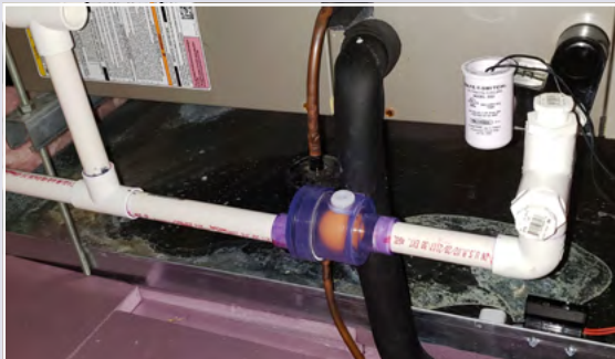
RLC-Series negative pressure trap replaced a leaking standard P-Trap that didn't have enough height to function properly.
