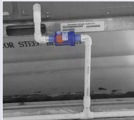
N-Series commercial rooftop negative pressure installation.
