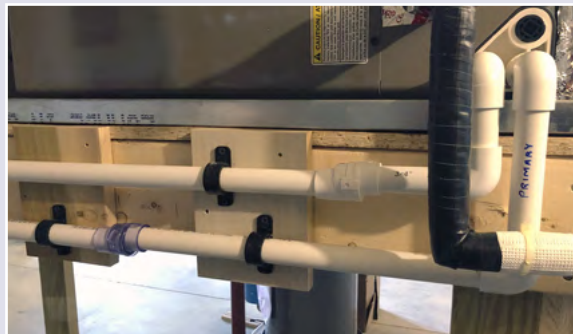
FCN-Series negative pressure commercial installation, an Air-Trap on both the main condensate drain pan line and secondary pan line.
