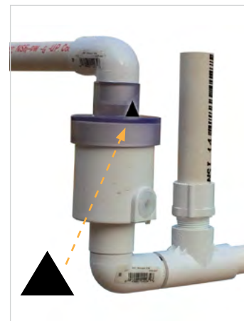
Figure 4 - Installation of a Vertical Vent Pipe installed directly downstream of a positive pressure trap to prevent a suction pressure that could develop depending upon the length of drainpipe, the diameter, and the water flow rate.
