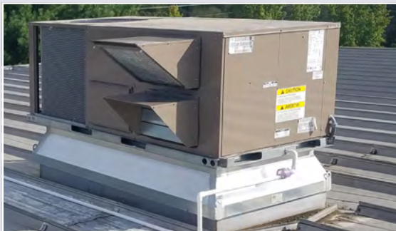
RLC-Series negative pressure commercial rooftop installation.
