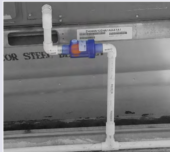
N-Series commercial rooftop negative pressure installation.
