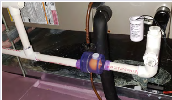
RLC-Series negative pressure trap replaced a leaking standard P-Trap that didn't have enough height to function properly.
