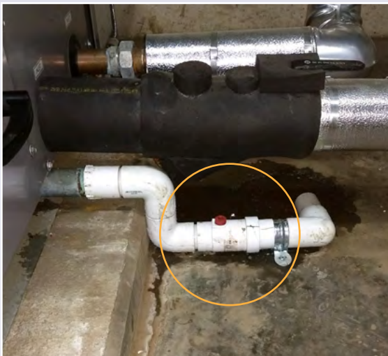
N-Series, commercial mechanical room negative pressure installation.
