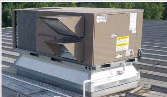
RLC-Series negative pressure commercial rooftop installation.
