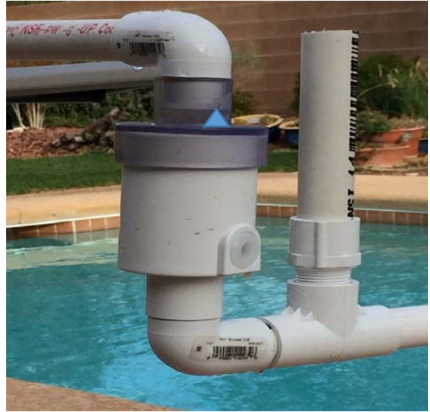
Figure 4: Installation of a Vertical Vent Pipe installed directly downstream of a positive pressure trap to prevent a suction pressure that could develop depending upon the length of drainpipe, the diameter, and the water flow rate.
