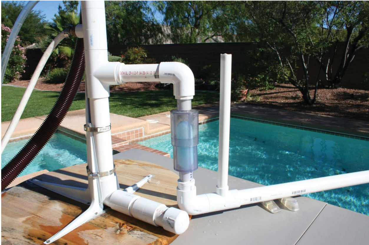
Figure 6 Positive Pressure HVAC Air-Trap undergoing tests at the Des Champs Technologies Las Vegas, NV test facility. Testing videos showing the operation of the trap are viewable at www.deschampstechnologies.com , then go to P-Series and then to P-Series YouTube Presentation
