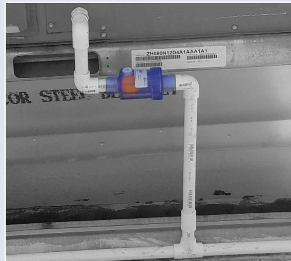
N-Series commercial rooftop negative pressure installation.
