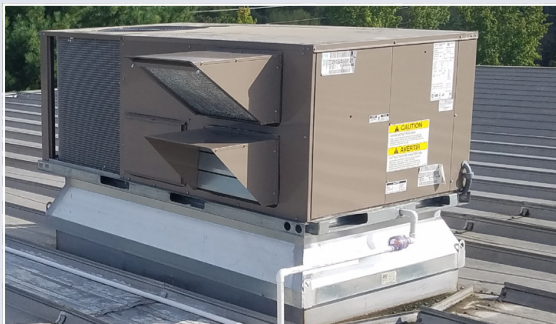
RLC-Series negative pressure commercial rooftop installation.
