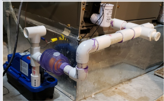
Attic residential RLC-Series negative pressure installation in combination with condensate pump.
