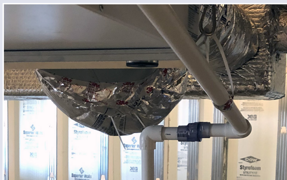
FCN-Series indoor commercial installation in negative pressure orientation.
