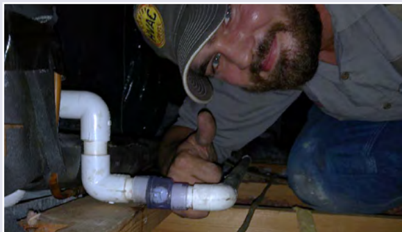
FCN-Series indoor residential attic install, negative pressure orientation. Tight space no problem, all thumbs up from the technician!
