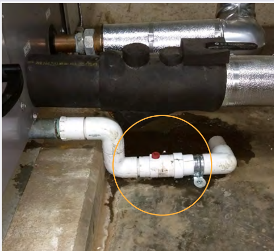
N-Series, commercial mechanical room negative pressure installation.
