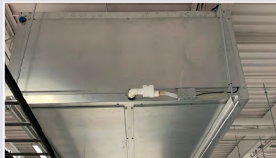
RLC Series negative pressure installation in a data center facility.
